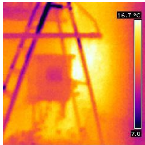
Outdoor energy meter producing heat
