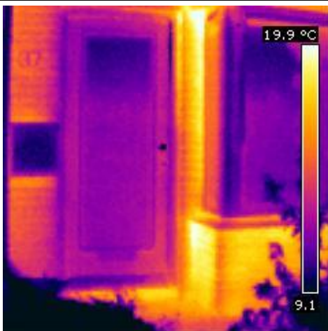
Poor thermal connection façade and bay
